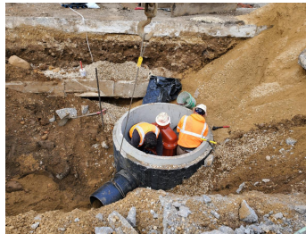
Water main valve vault
